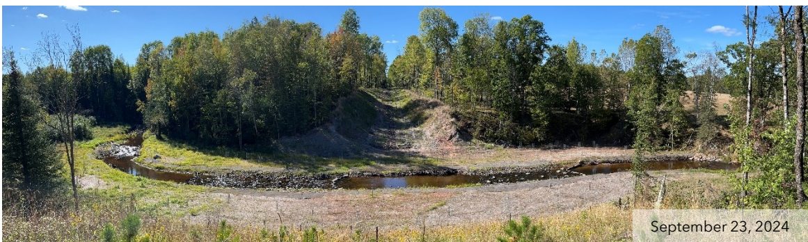
Figure 4. Nebagamon Creek abandoned railroad grade excavation site facing west. (Photo credits: Wisconsin DNR)
